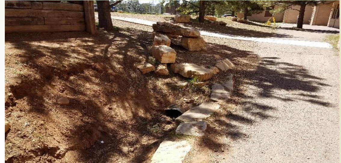
FIGURE 5: SEDIMENT IN CULVERT B [3]
