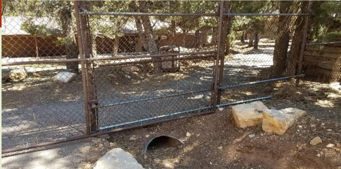
FIGURE 4: SEDIMENT IN CULVERT A [3]
