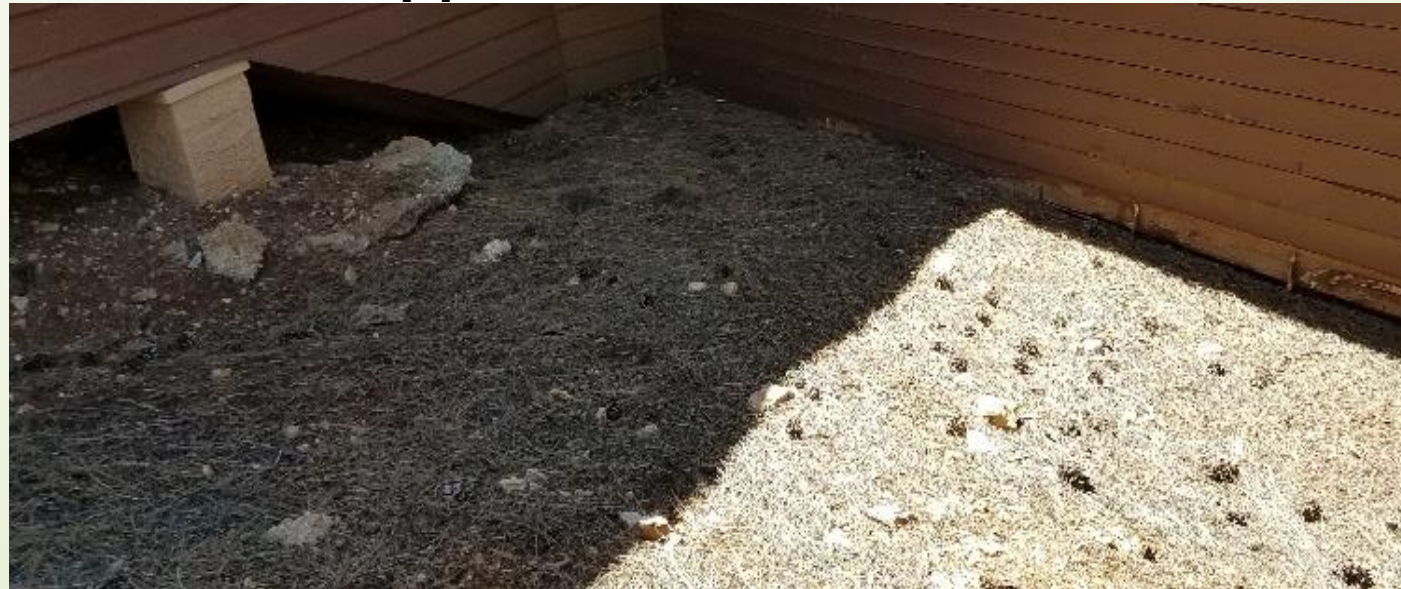
FIGURE 6: AREA OF SURFACE FLOW WITH STRUCTURE FOUNDATION IN PATH [3]
